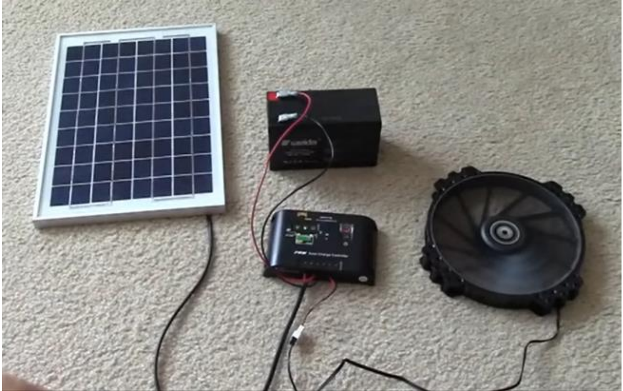
Off grid: charge controller 6 terminals of solar battery load
